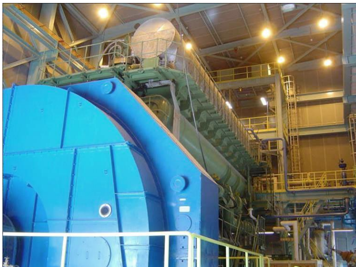
View of the existing engine at the Chios plant
