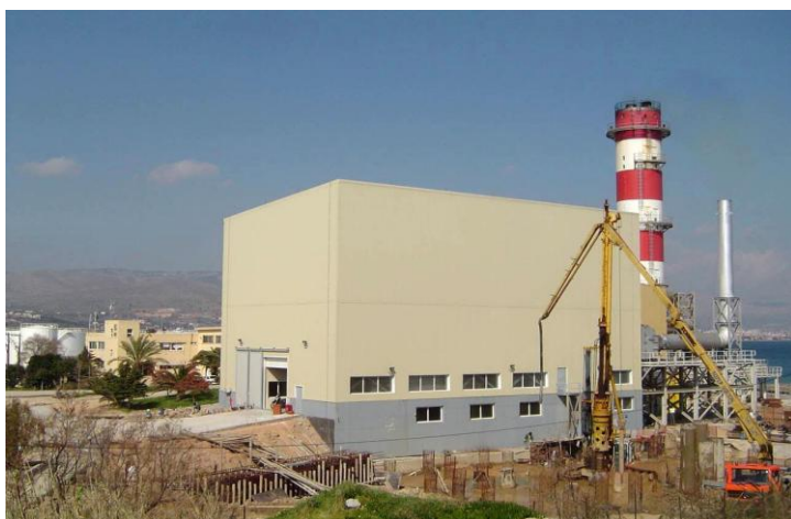
External view of the Chios power plant
